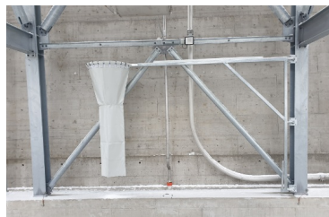
Filling pipe of the silo plant in Zernez
