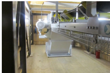
Loading facility of the grit silo plant
