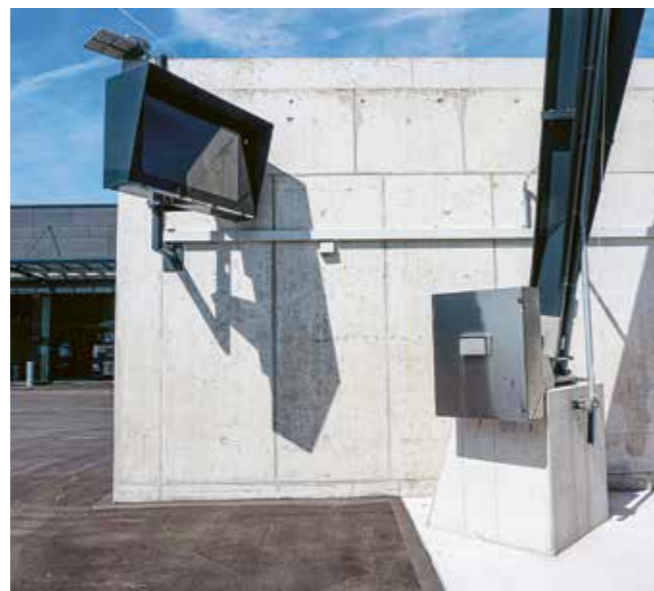
↑ Complete winter services facility with timber silos and brine facility. ↶ The hoppers are controlled automatically via the top-class automatic system. ← The screen helps drivers monitor the filling process.
